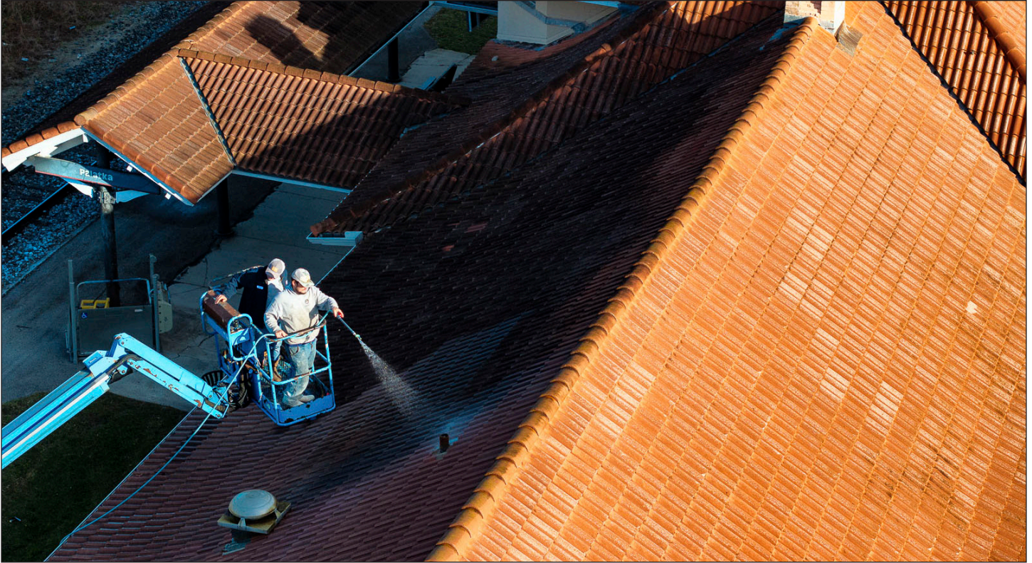
Contractors working for the City of Palatka pressure washed the roof of the city-owned railroad station last week. The City's Code Enforcement Department cited the City because the roof was dirty and did not meet code.
